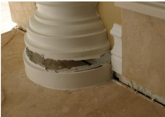
Fig.1(a,b,c): cracks identified by Visual Inspection
