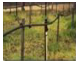
(c): Sprinkler System
